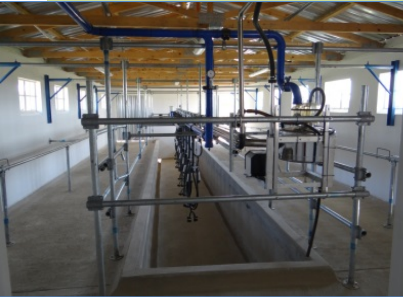
Diyatalawa Milking Equipment (FS)
