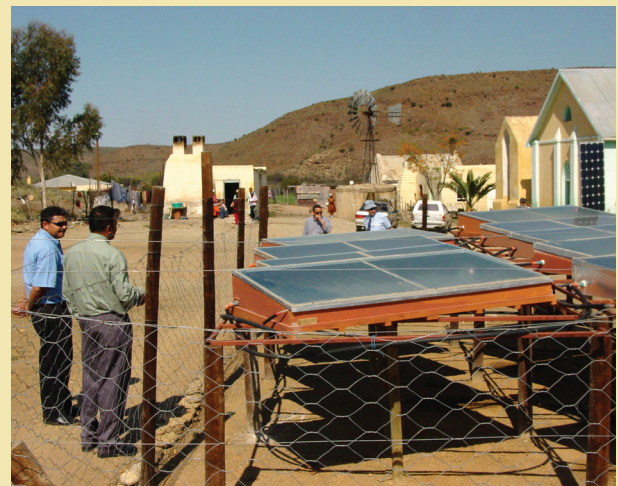
Solar panels are used to generate renewable energy.
