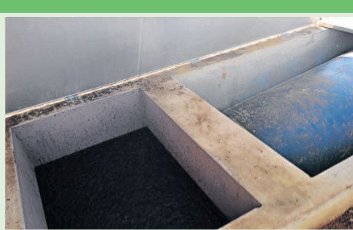
Balloon Biogas system installed at the Sharpeville Primary and Tygerkloof High Schools with bio fertiliser produced.
