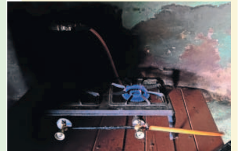
Fully functional biogas system in Mpfuneko.
