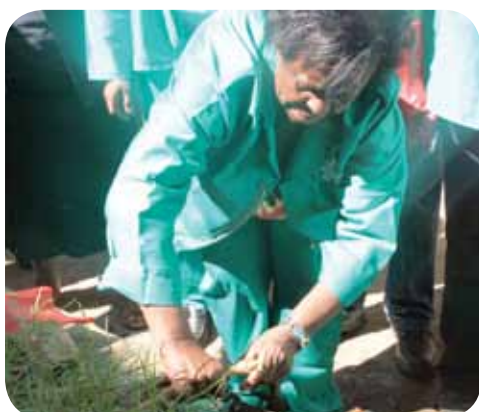
Fixing: Former Deputy Minister Mabudafhasi at uMsobomvu Primary School fixing one of the leaking taps in the school.
