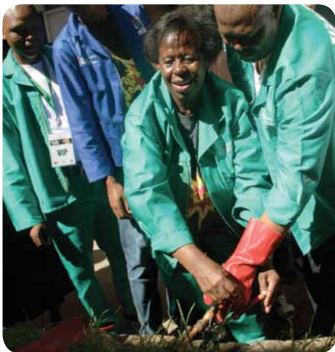
Former Deputy Minister of Water and Environmental Affairs, Mabudafhasi with the Mayor of Mquma Municipality Councillor Ginjana fixing taps at the uMsobomvu Primary School as part of the War on Leaks and War on Waste project launches.
