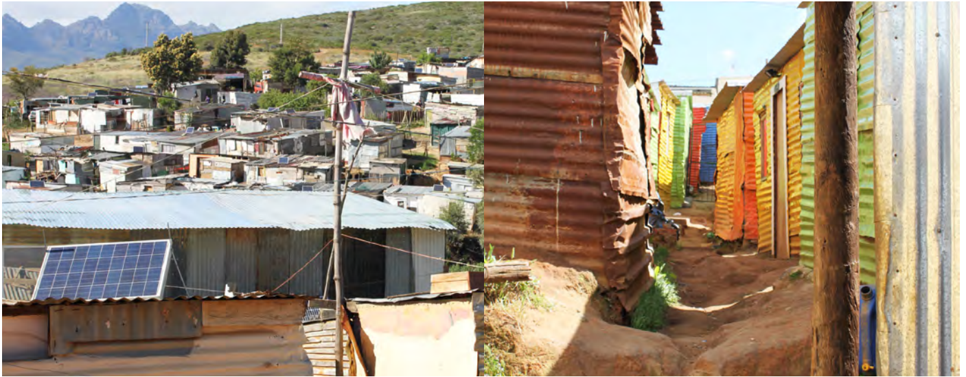
Above: The iShack Project installs off-grid Solar Home Systems in the shacks of residents who voluntarily sign up for the service.
