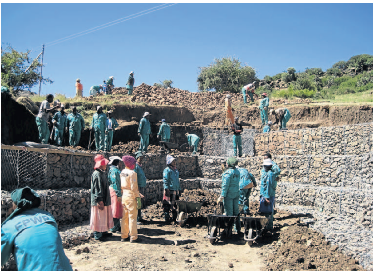
Land care and unemployment amongst poor and unskilled South Africans, are amongst the matters addressed by government's cross-cutting Expanded Public Works Programme
