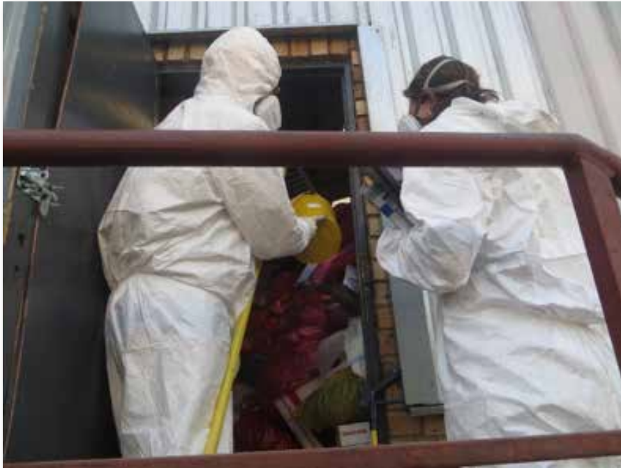
Picture: photos taken at the initial site inspection.
