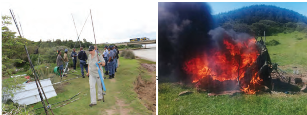
Fish River operation in Eastern Cape, illegal structures demolished and illegal fishing activities dealt with.
